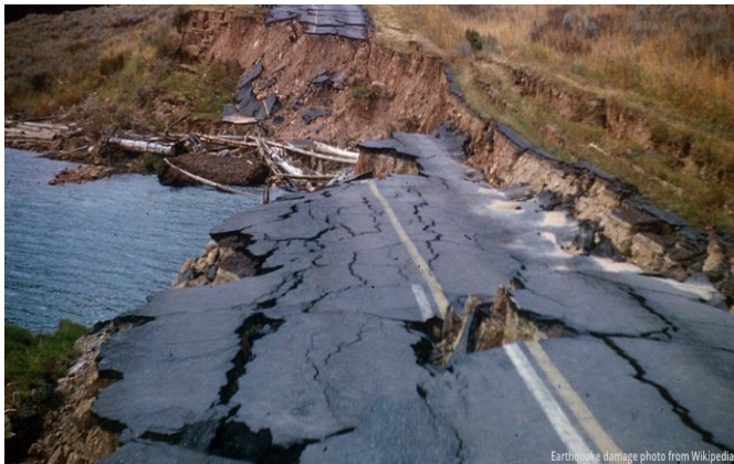
Earthquake damage photo from Wikipedia
